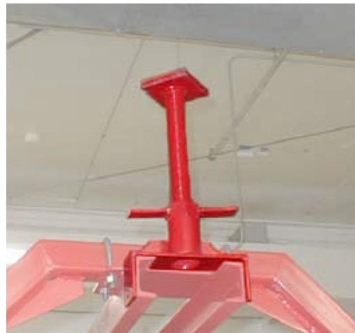
Ceiling Brace (PT-3)
