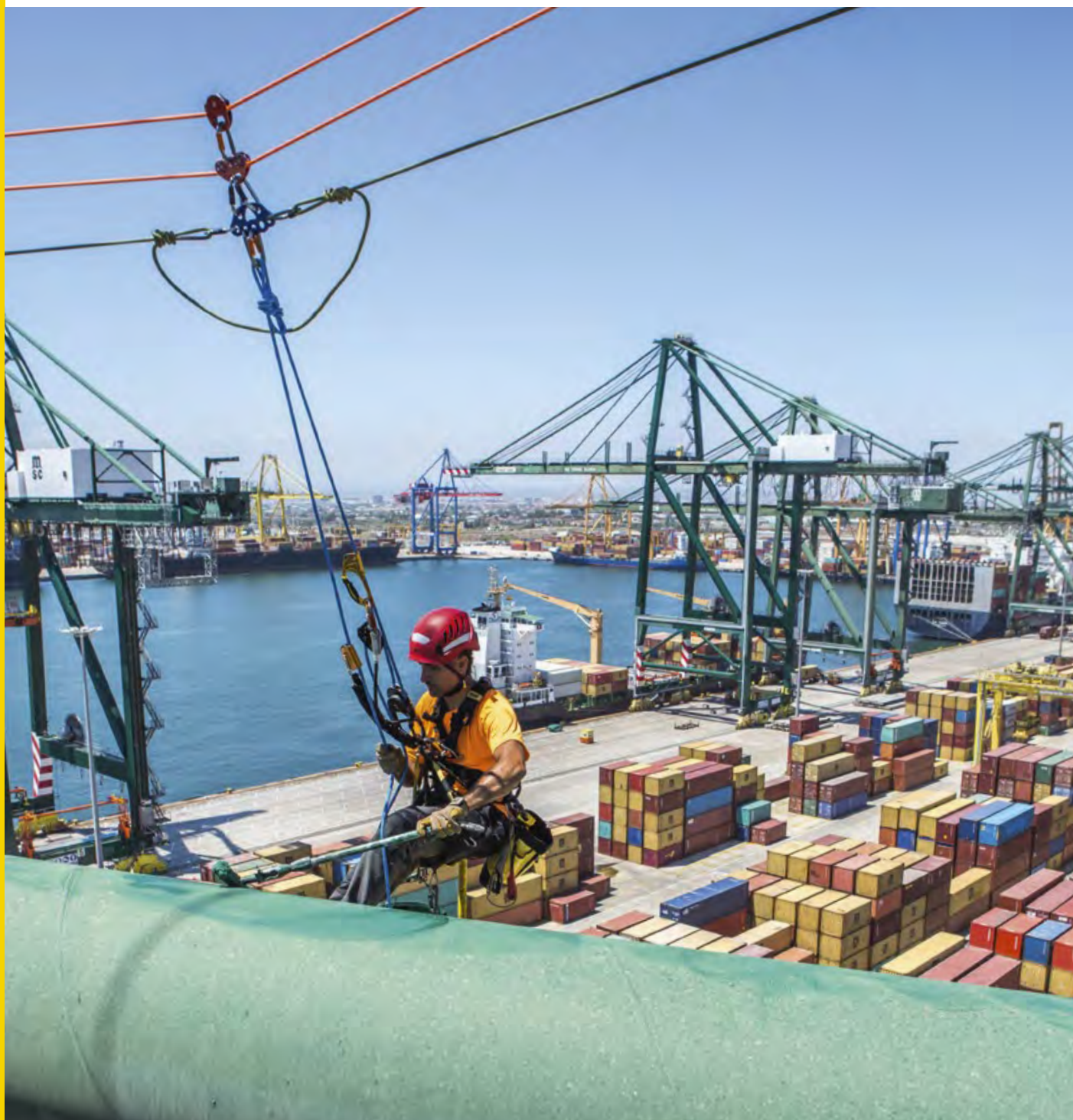
Paint job for the cranes of the merchant harbor of Valencia, Spain. © Petzl - Jan Novak photography - Vertice Vertical™
